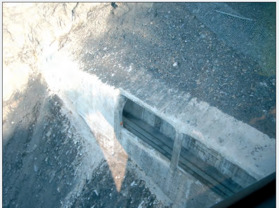
Figure 15 - After the structure had been strengthened, the talus recovered its original form.
